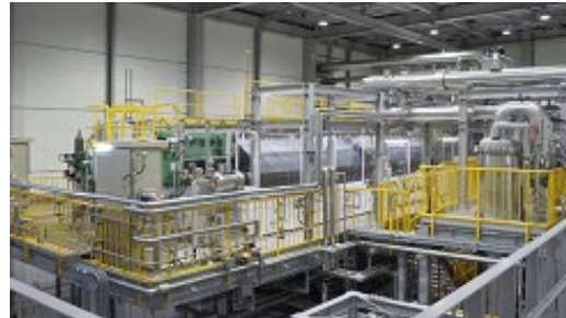
Hydrogen Production through Water Electrolysis Using Power from Renewables
