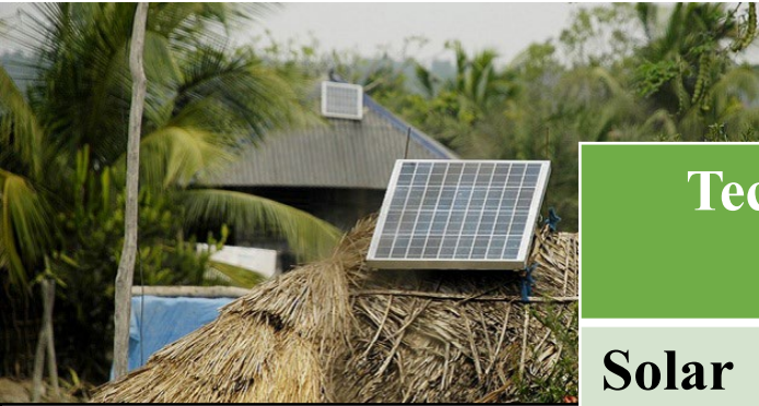
Solar Home System
