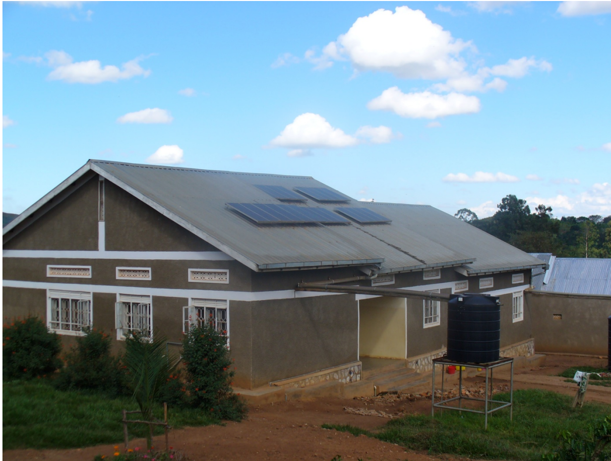
Solar PV Systems installed at a Health Centre
